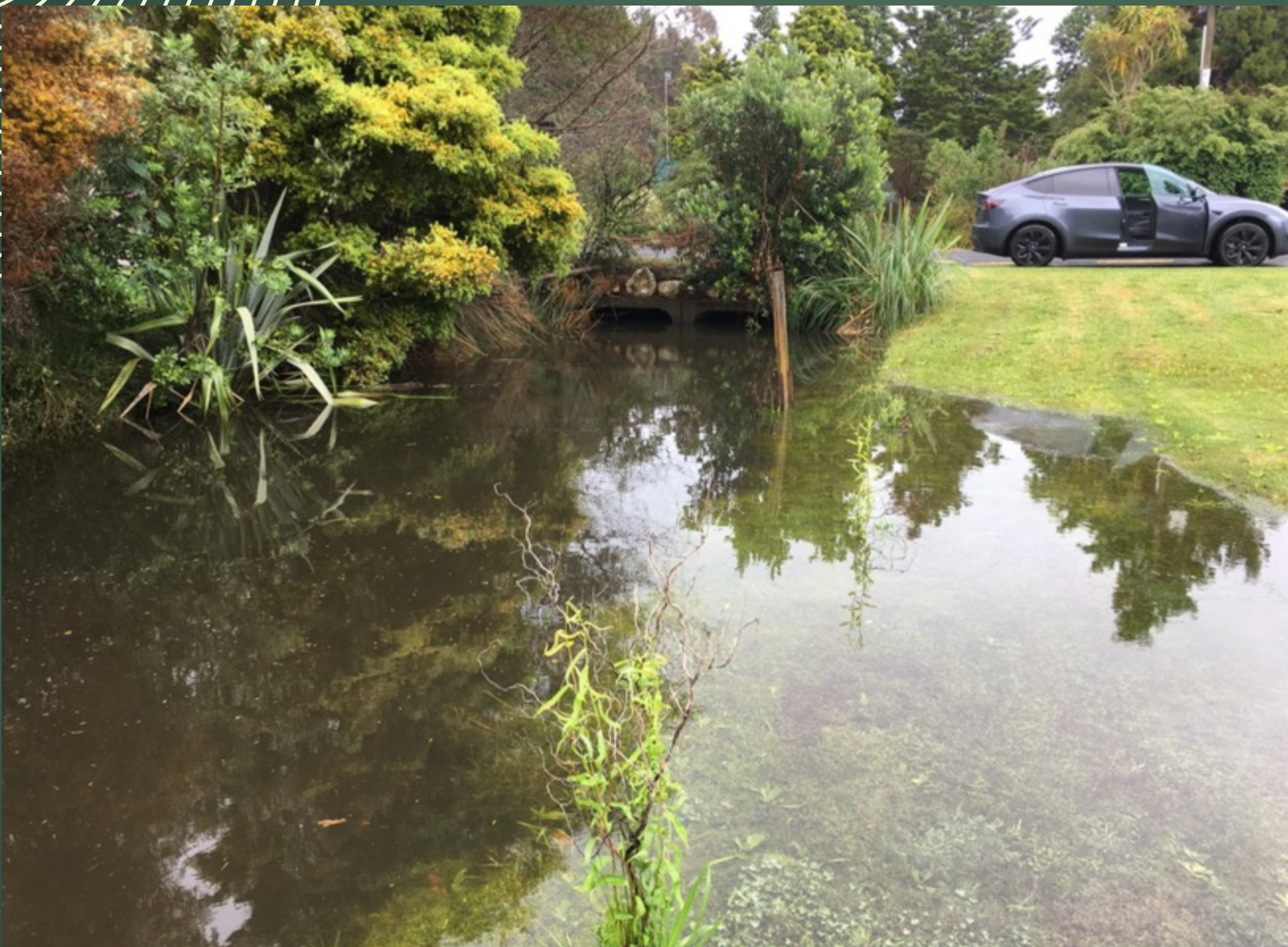
Rees Ave culvert - 2.1 m High tide - post a dry period, tidal flow upstream
